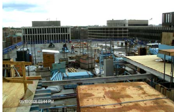
Figure 6 View of 13th floor west pour (area 2) from 14th floor east framing, 2 days after 13th floor east pour (area 1)
