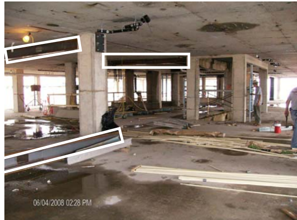
Figure 15 Structural steel reinforcing around stairs and elevators. Piece on lower left to be installed
